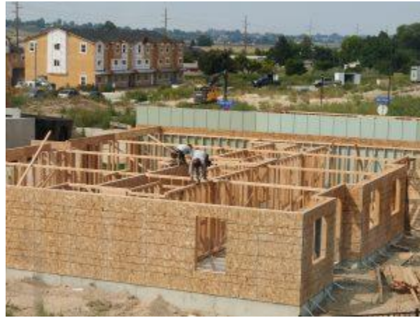
Construction of the expansion of The Franklin at Ten Mile. Photo by Sharon Fisher
